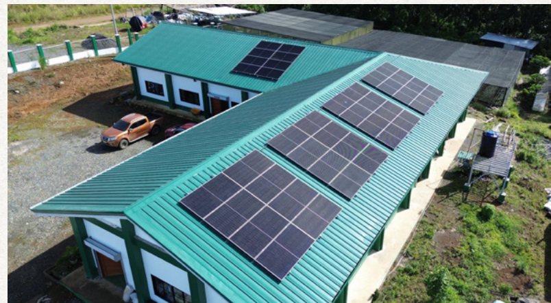
Solar and batteries on the cooperative's own roof, installed with support from the Peace and Equity Foundation's PURE initiative. Image courtesy of the Peace and Equity Foundation.
